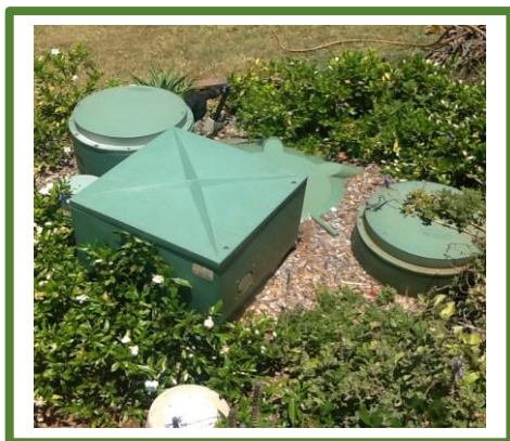
Sewage Treatment system, utilising the Fully Aerobic Activated Sludge technology
