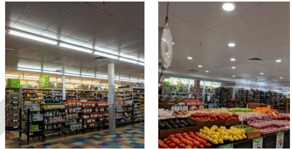
Program in place to gradually replace T8 fluoro tubes with energy efficient LEDs downlights
